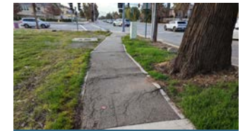
Sidewalk near elementary school buckling due to adjacent tree roots. ↴ Grapeland Elementary School
