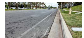
Bicycle lane lacks buffer from vehicles and needs maintenance.
