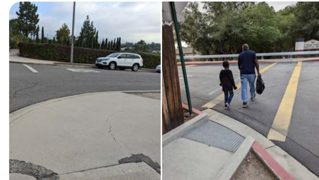
Pedestrian facilities around Valle Vista Elementary can be enhanced with high visibility crosswalk striping, curb ramps, and curb extensions
