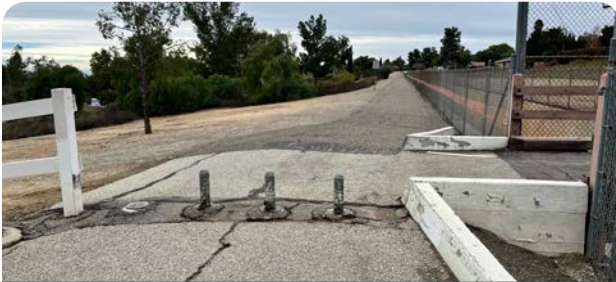
Trail access locations at Demens Creek Trail would benefit from trail crossing improvements.
