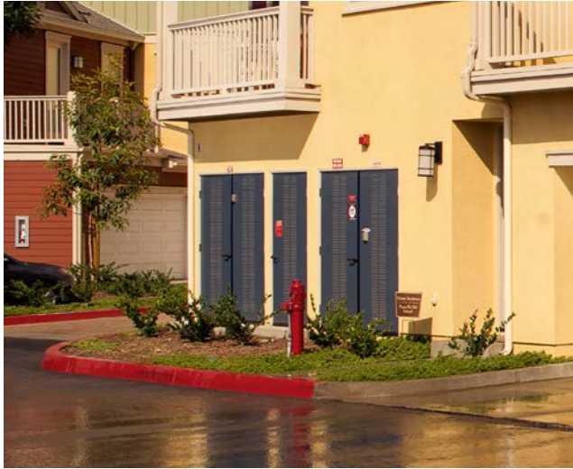
Utility cabinets integrated in architecture
